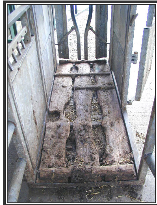
Figure 5.23.: An example of a badly worn wooden floor in a crush.
